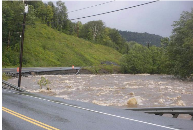
This photo shows the real connection of river and road during TS Irene, as the river reclaims its floodplain, edging in on the road. Photo courtesy of wilmingtonvtfloorelief.com .
